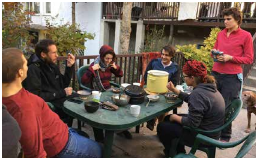
Builders - members of the cooperative - and allies enjoy lunch break while renovating the first rental cooperative house in Budapest. Credit: MOBA Housing Network
