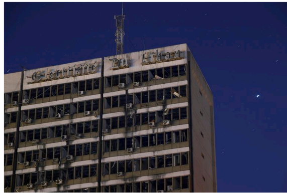
Fig. 1. Lebanon's Electricity Company (EDL) headquarters in the aftermath of an explosion at the port area in Beirut, Lebanon, August 16. REUTERS/Hannah McKay.
