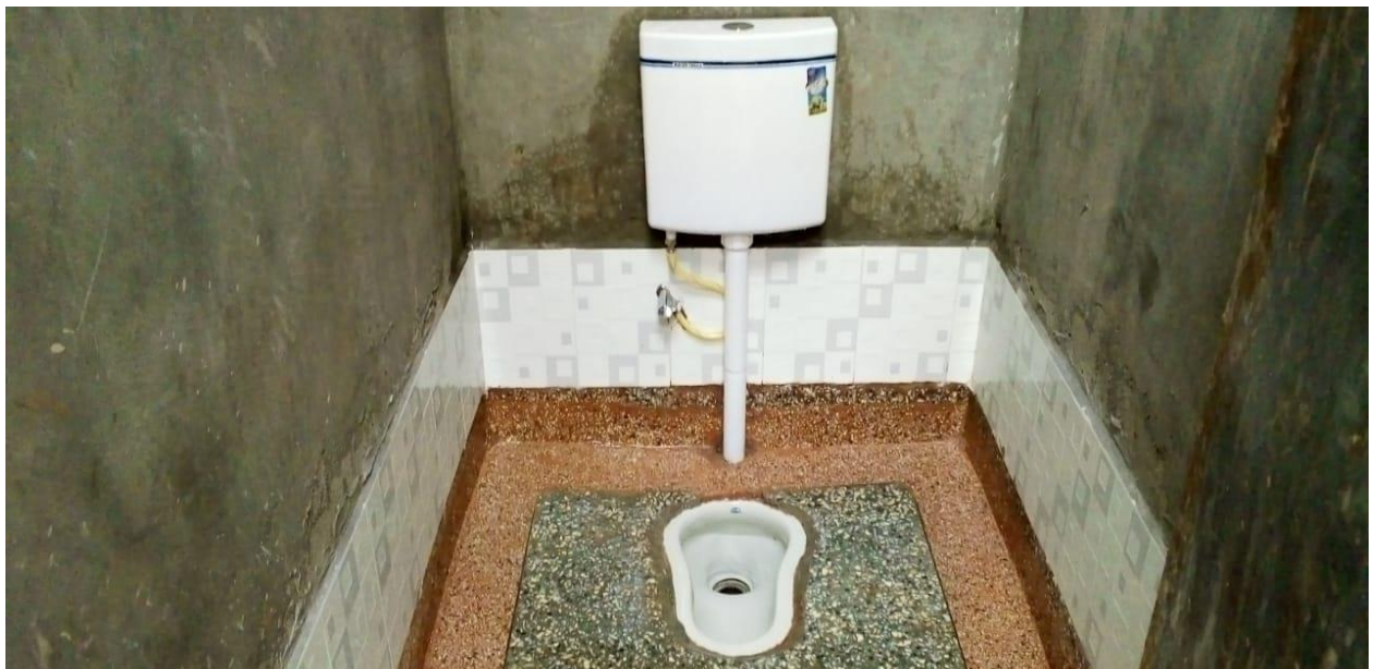
Figure 43: An example of pour flush Sanitation technology provisioned by HOP in Mukuyu primary school
