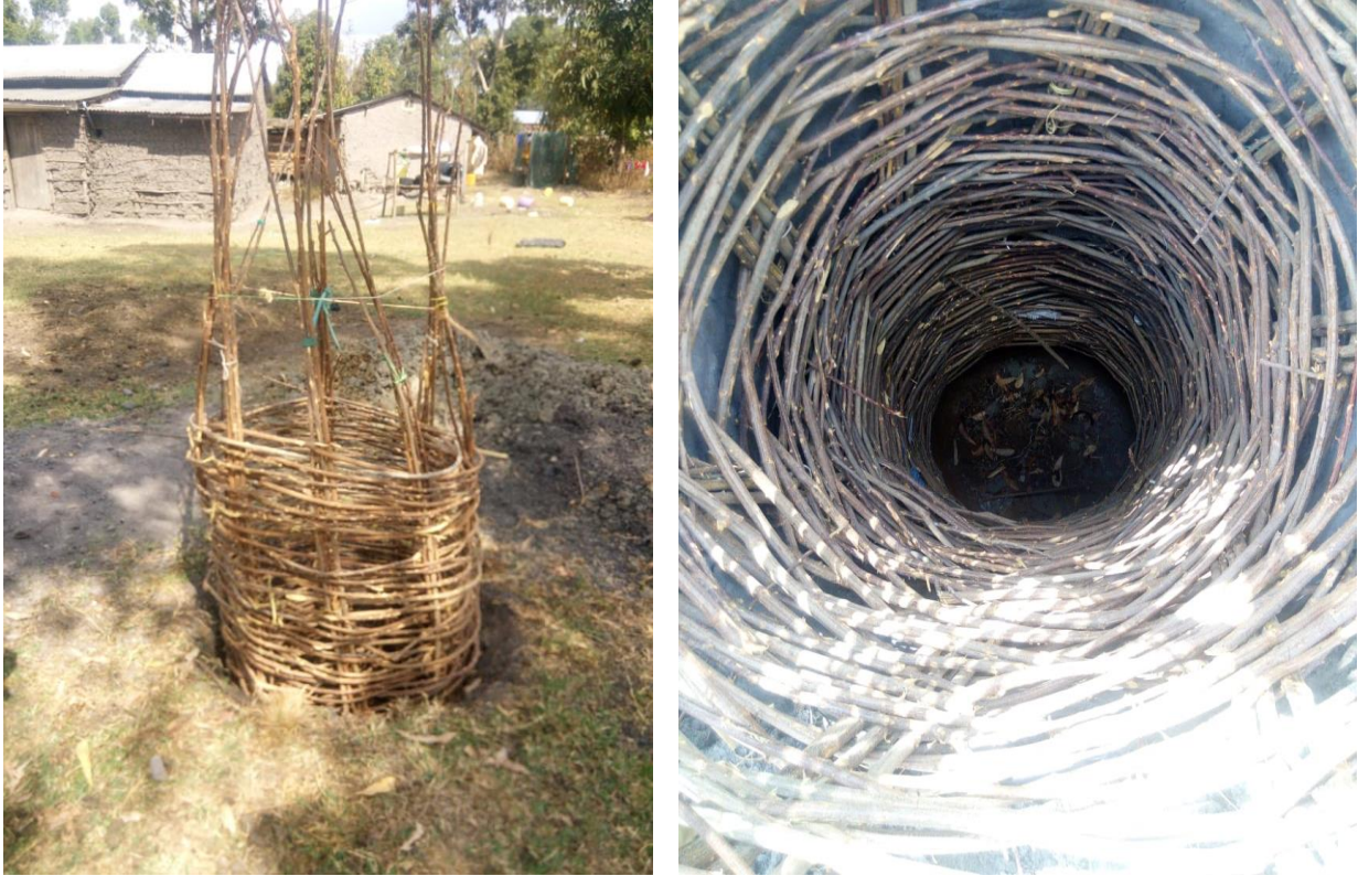
Figure 36: Adapted pits structure used to tackle loose soil in the region that used to be the main cause of pit collapsing
