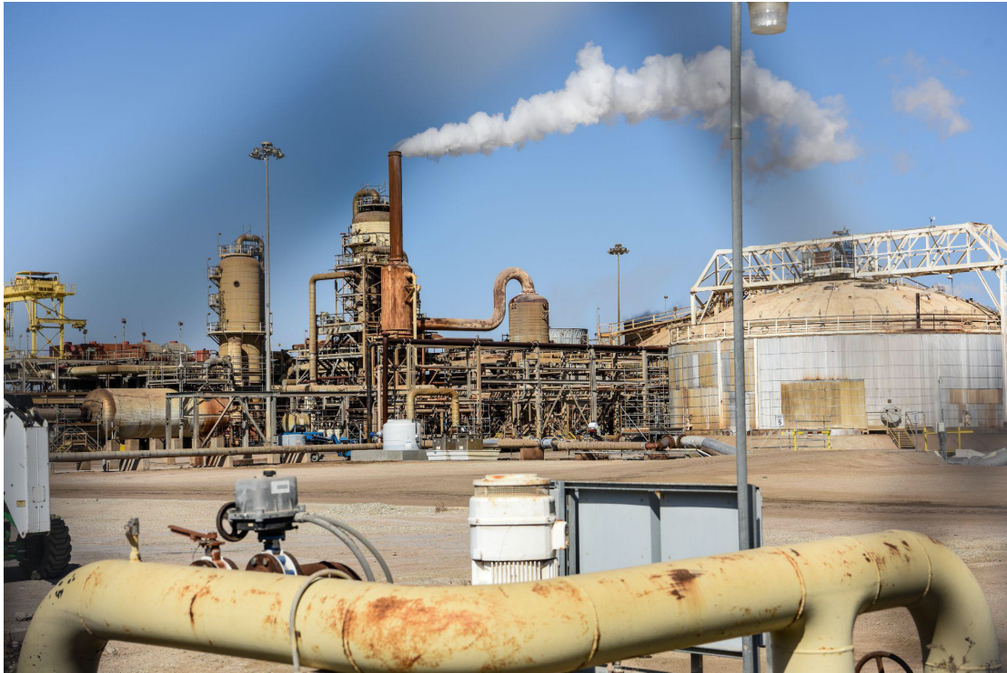
Figure 4: CalEnergy Geothermal Plant near the southern shore of the Salton Sea (Geoffrey James Britton, 2021)
